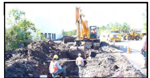
In this photo (bottom right), Johnson-Davis of Lantana does the water, sewer, and drainage infrastructure work on the project, with pipe and fittings supplied by Sun Pipe.
