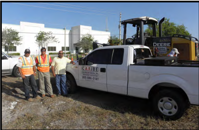
(RIGHT PHOTO) Here the Caribe crew trenches for the 12" line that will run along the west side of 120th Avenue, from Wiles to Sample Road.
